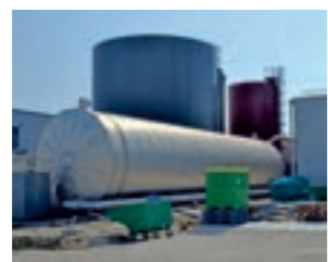
Hot water storage
